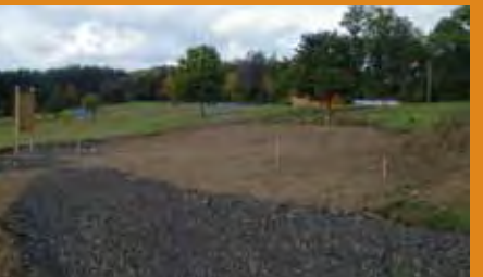
Through a grant from Recreation Equipment Incorporated and funds from PPF, the Friends of Shawnee have started the construction of a new handicapped accessible amphitheater at Shawnee State Park (unfinished project.)
