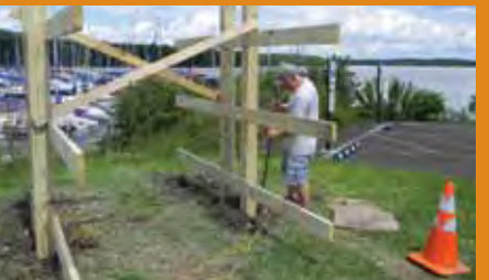
The Friends of Nockamixon State Park received a matching grant to construct two small boat/kayak racks and a mast hoist at Nockamixon Marina.
