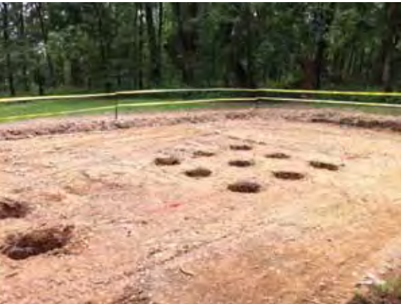
The building of the new playground at Samuel Lewis State Park in memory of Leah Vogel.
