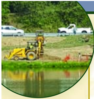
Site work has started on the ADA launch at Little Buffalo State Park.
